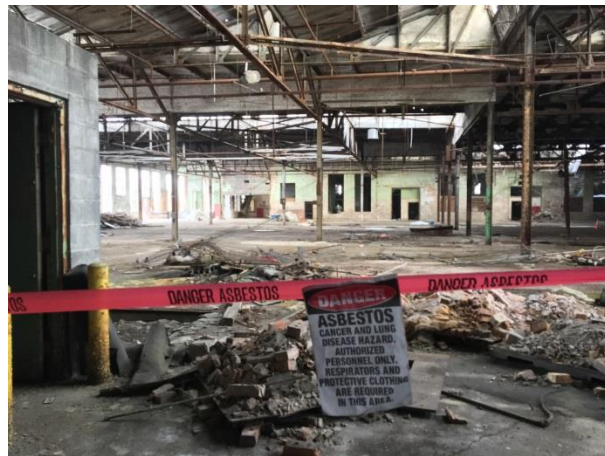
An area of the main factory floor at the former H.K. Porter site is cordoned off in preparation for United States Environmental Agency contractors to abate asbestos and other hazardous materials during an earlier phase of the cleanup.
