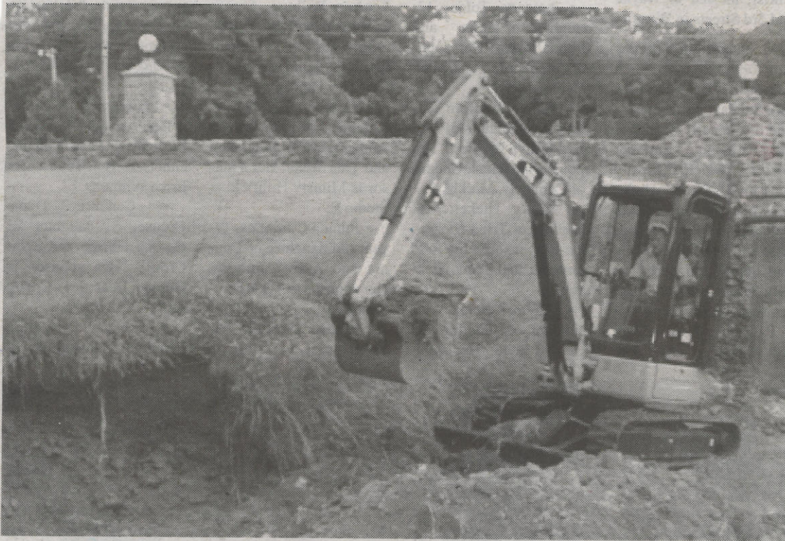
Ray Starr, owner of Ray Starr Masonry and Roof Restoration, removes the old retaining wall on the south side of West Park Drive at Sunken Gardens in Huntington on Monday, June 21. The wall demolition is part of a larger project to restore the masonry in the park. Photo by Matt Murphy.
